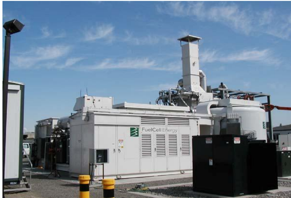
Molten carbonate fuel cell at King County South Treatment Plant, Seattle, WA. (Photo: King County)
