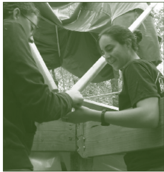
CEP Students Aspen Price (left) and Elizabeth Pratt fastening wall poles to the floor frame on a Woodframe Yome.
