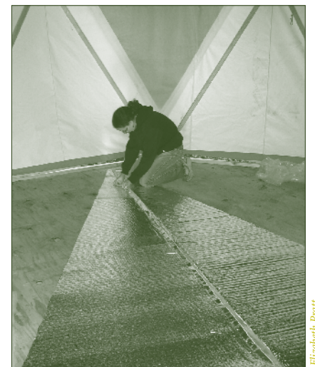
Aspen Price taping together panels of roof insulation for a Woodframe Yome
