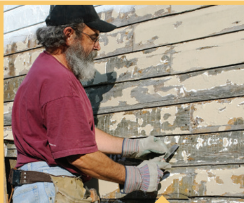
⊘ Unsafe home repair
