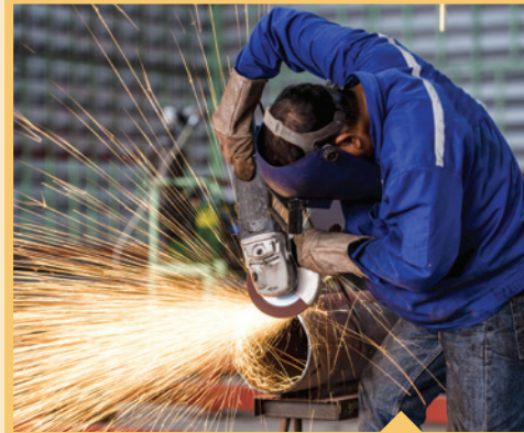
⊘ Workers exposed to lead
