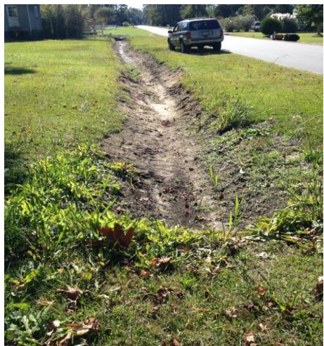
Ground excavation for placement of new water line. Photo credit Karen Villeda
